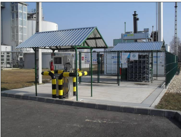
Biometan tank station
